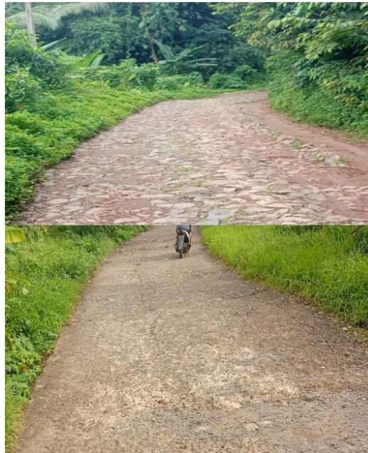
Figure 1. Road damage that needs to be repaired (Source: Personal documentation)
